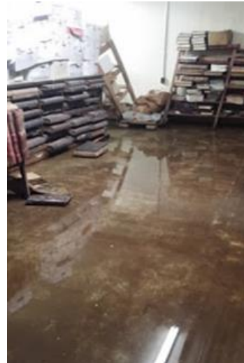
Standing water in the basement
